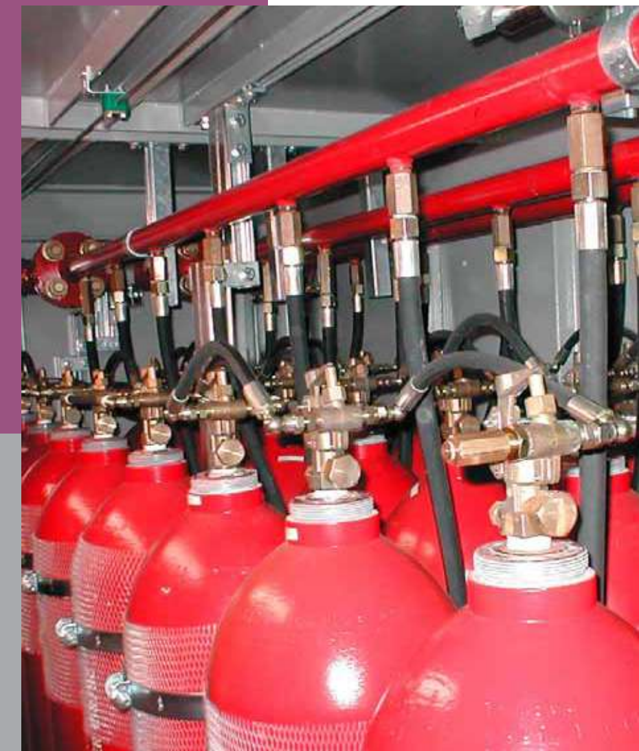
CO 2 Snuffing System Offshore Nigeria
