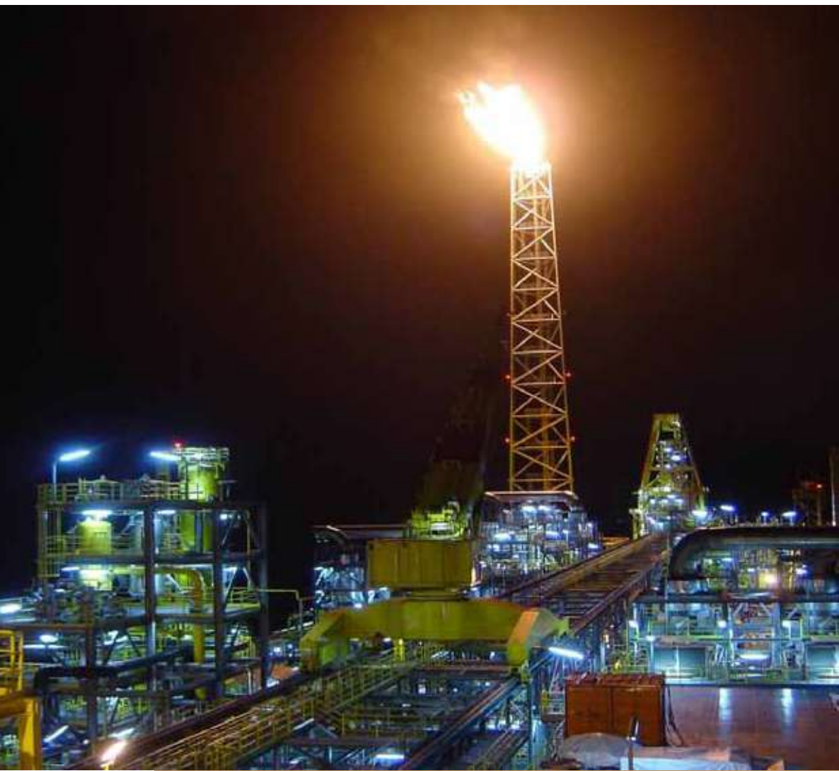
CSF-6-8-HL-14 HP/LP Flare Tip FPSO offshore Nigeria
