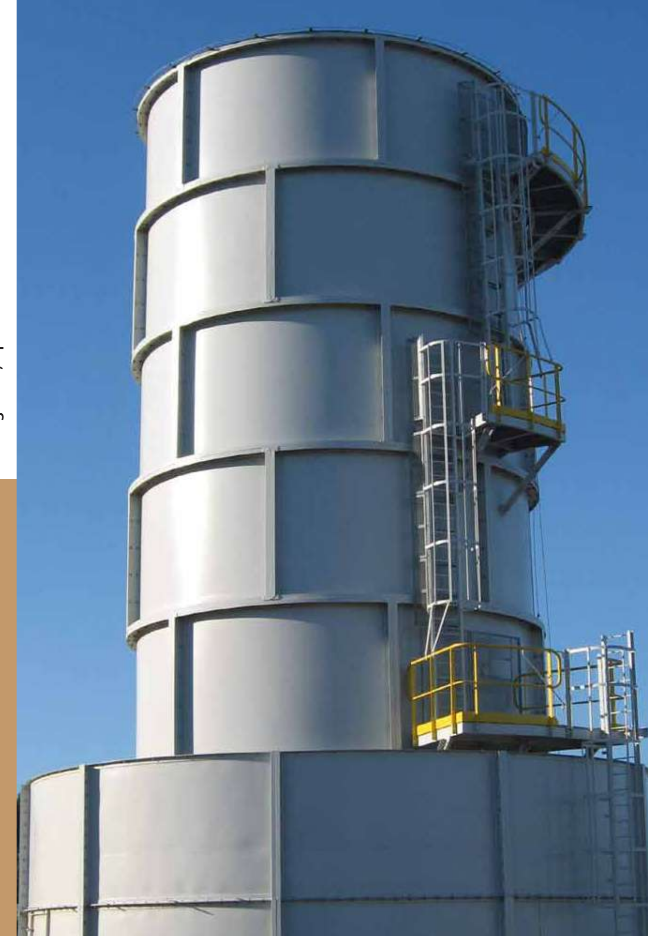
15t/h Enclosed Ground Flare Mugardos, Spain
