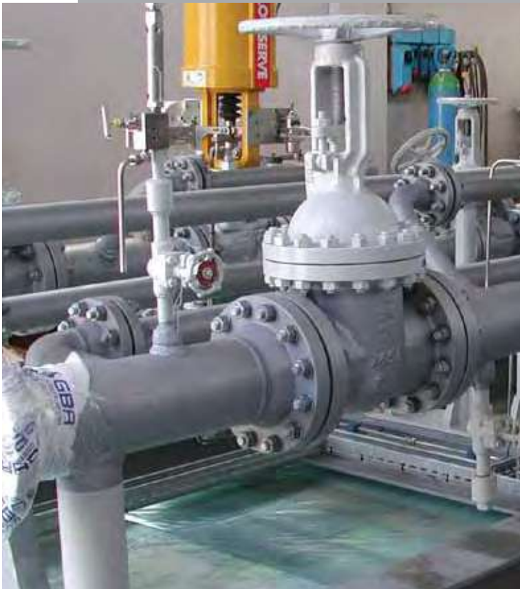
Steam Control Skid Petrochemical plant UAE
