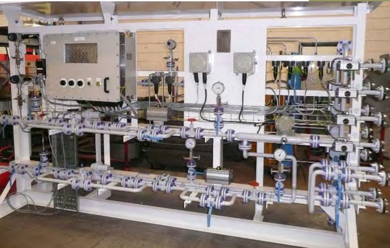
Flame Front Generator Ignition System (FFG) with fuel gas control Onshore gas terminal project, Turkmenistan
