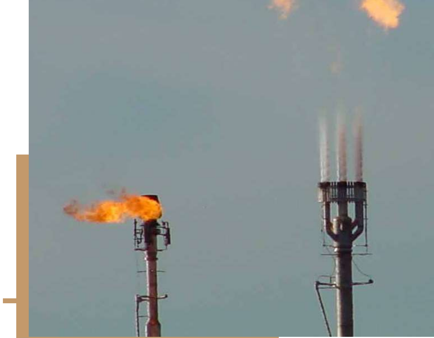
CSF-7-14 Flare Tip Gas plant Alaska
