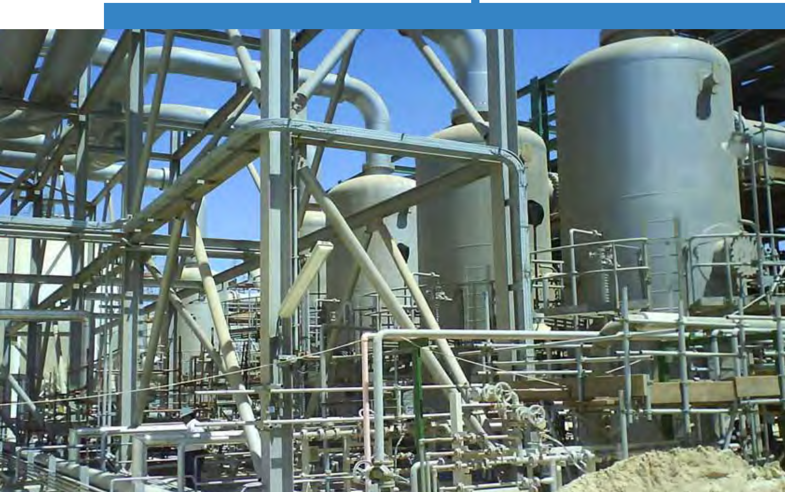
Water Seal Drums Petrochemical plant, Saudi Arabia
